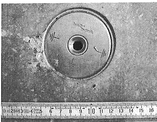
Illustration 2: Grounding penetration passage HEA-IS-M12/100, concrete trough inner side
